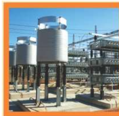
Harmonic Filter Bank
