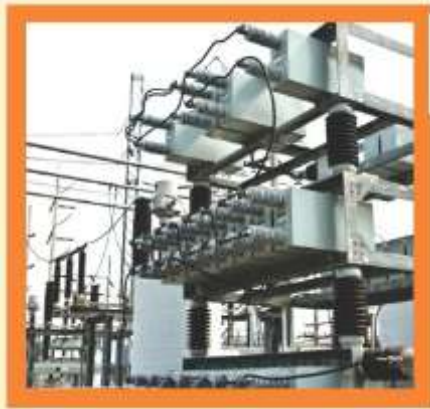
Open Rack Substation Bank
