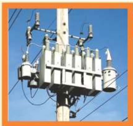
M.V. Pole Mounted Capacitor Banks
