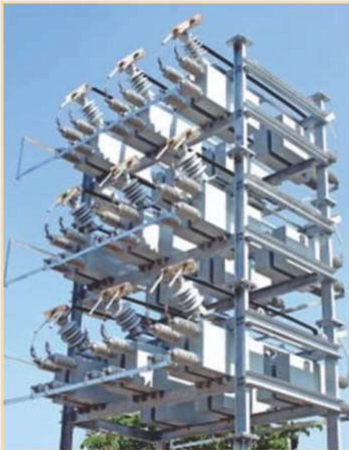
Scope Supply of 33 KV Fixed Type Structure Mounted Capacitor Bank
